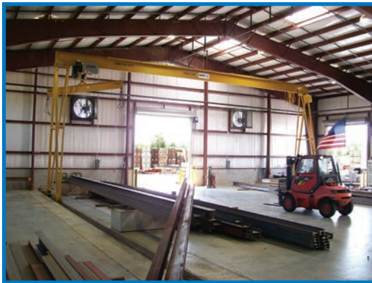
A Spanco Motorized 7.5-ton PF-Series Gantry Crane used to move truckloads of long steel beams at a building material supply center
