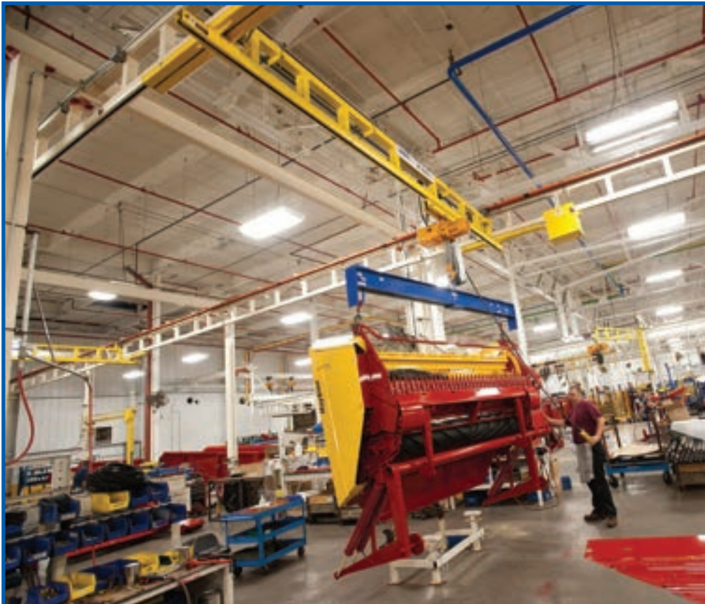
An agricultural equipment manufacturing operation using a freestanding workstation bridge crane with runways supported by steel columns.
