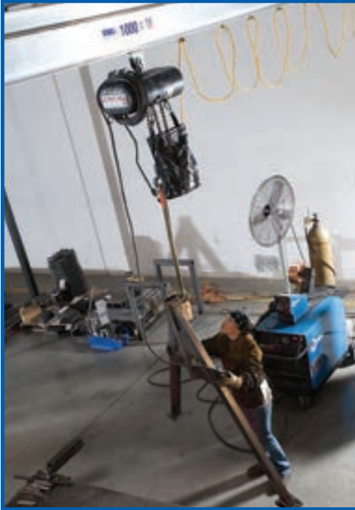
A worker uses a 1,000-pound capacity Spanco Alu-Track Bridge Crane to position product in her work area.
